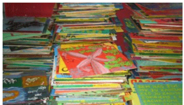
The mammoth task of 1000's of tiles that need to be fixed into place!
