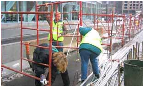
The construction of the scaffolding to keep the huge climate mosaic in place.
