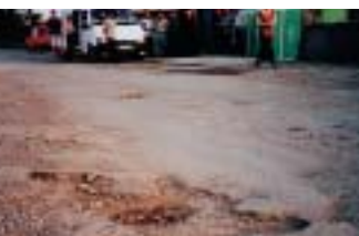
Agtagla village – road damage (Greg Muttitt/Bank Information Center)
